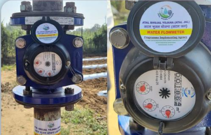
>3 lakh data entries recorded through Water flow meters installed on wells
